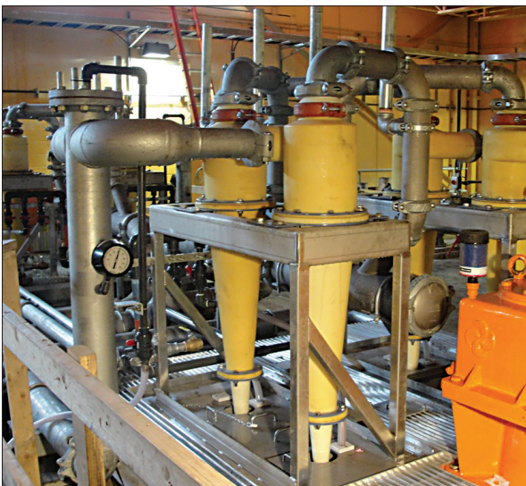
Hydrocyclone set-up for microsand recirculation within the Actiflo process.
