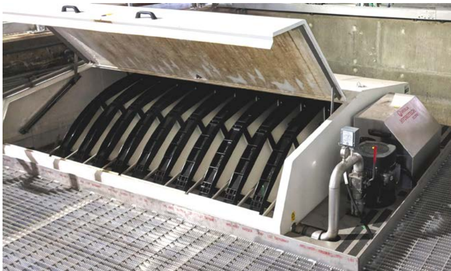
The compactness of the disc filters allowed them to fit in the Banff WWTP's existing sand filter basins and allowed for future expansion if needed.
