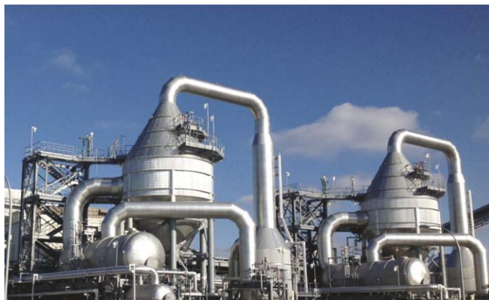
Figure 4. Thermal solutions, such as the one pictured, help large producers achieve better economies of scale for water treatment needs. Implemented through multi-stage evaporation, thermal systems often achieve 80 – 90% water recovery. However, when crystallisers are incorporated to concentrate solutions beyond salt saturation levels, the operation precipitates dry solids reaching zero-liquid discharge, with water recoveries topping nearly 100%.
